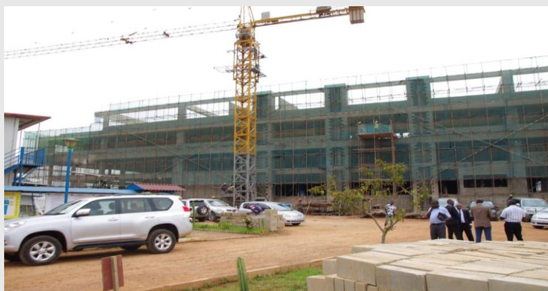
A view of the mid-level stages of the NMS warehouse construction works during a site visit by Ministry of Finance, Planning and Economic Development officials.
